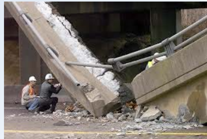
Collapse of structure due to extensive cracks
